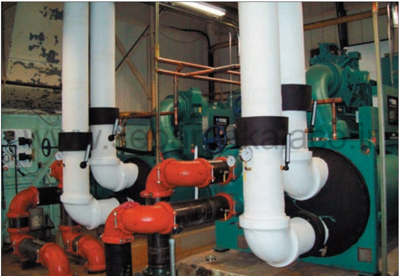
Gleason Cutting Tools installed a centralized chiling system to conserve energy and reduce shop floor costs (Courtesy of Gleason).
